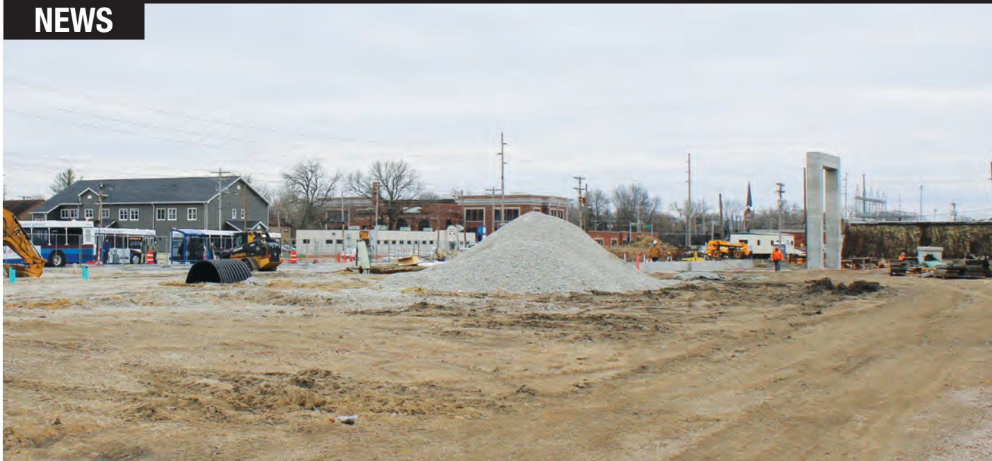
Site work has begun for the future Springfield-Sangamon County Transportation Center, and the county has asked the YMCA of Springfield to survey the community about interest in a potential second downtown branch in the center. PHOTO BY STACIE LEWIS
