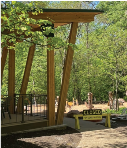
Construction is wrapping up on the new Children's Woodscape Garden, expected to open this summer.
